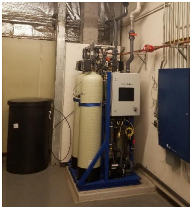
This water savings system is installed at the Lloyd D George Federal Courthouse in Las Vegas Nevada.
