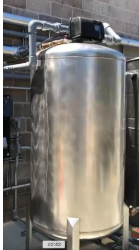
ApHinity CIO2 Installation in a major Hospital in California providing millions of gallons of water savings in the first months of operation
